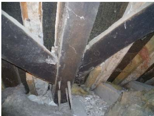
Photo 5: Smoke-blackened principal rafter and windbraces
